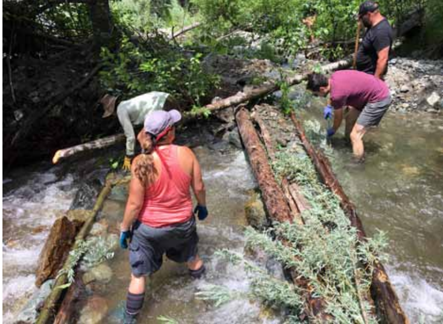
A joint training and workday building step-pools on Stanshaw Creek with the Karuk Tribe, MKWC, USFWS and SRRC
